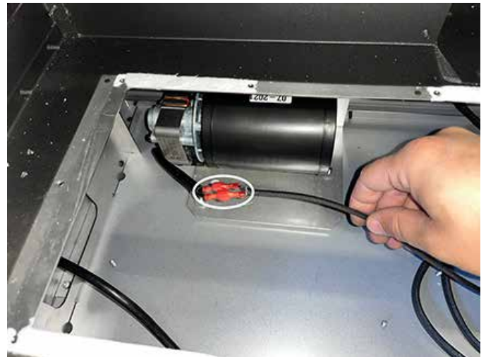
Figure 80: Blowers connected to wire harness
