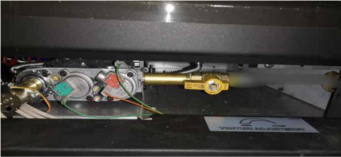
Figure 42: Z25 Valve and shut off.
