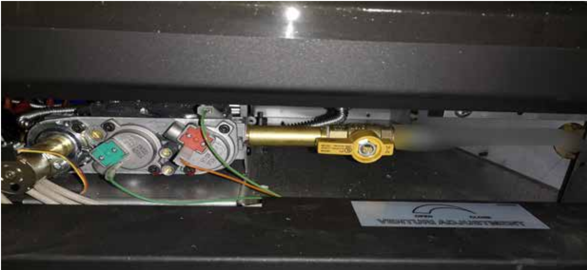
Figure 41: Z25 Valve and shut off.
